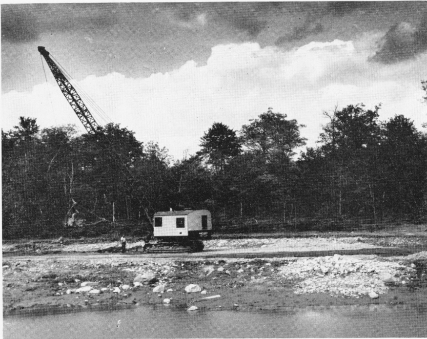
Against a background of trees and cloudy skies, the work of cleaning out the basin of the Brass Mill Pond was pictured. The mud and silt is being dredged out of the Pond in order that it will hold more, and a cooler body of water for use in Scovill manufacturing. The machine at work is a fifty-four-ton, 1½ yard, diesel-powered dragline shovel, with an eighty-foot boom. The bucket is capable of digging 135 feet from the machine, and of excavating from 1,200 to 1,600 cubic feet a ten-hour day.
